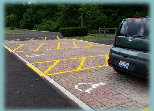
Permeable pavement reduces ice-build up and acts as a safety feature for handicapped parking stalls.
